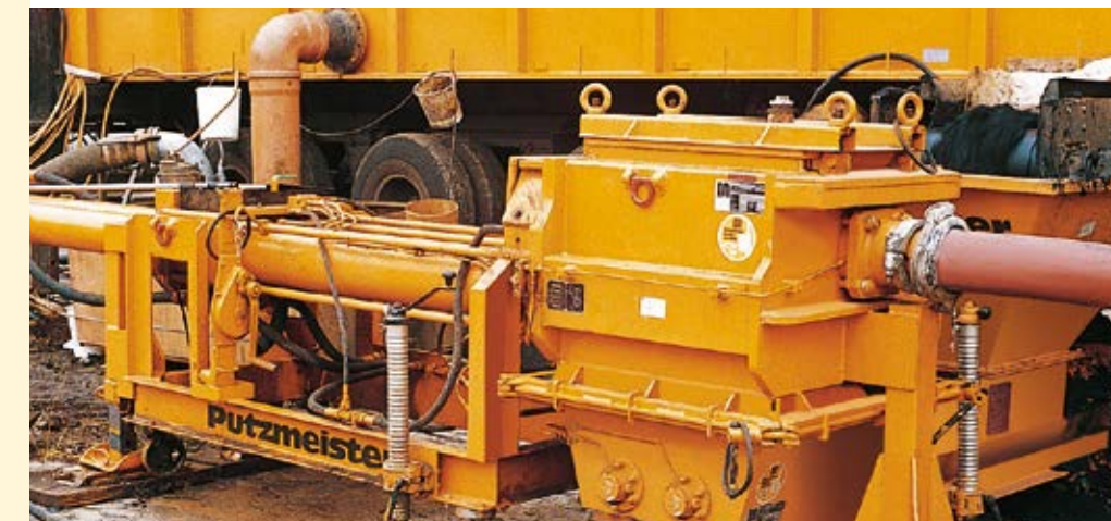
Mobile dewatering and pumping station
