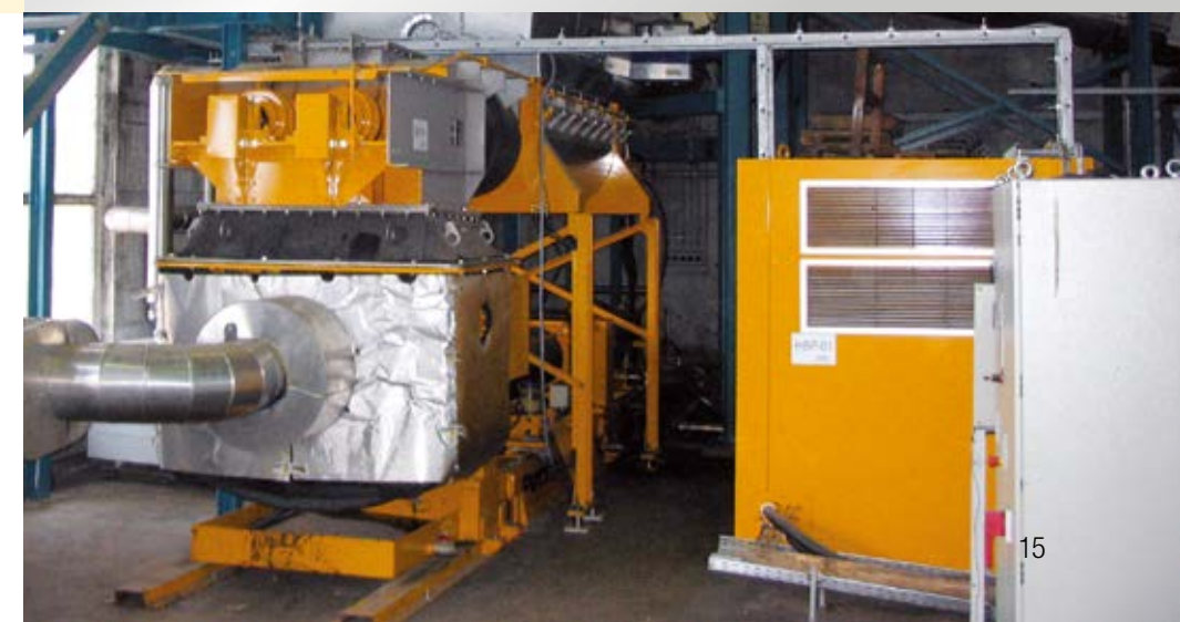
KOS 25100 with hydraulic power pack and twin-screw feeding device, transporting biomass to the fermentation tank
