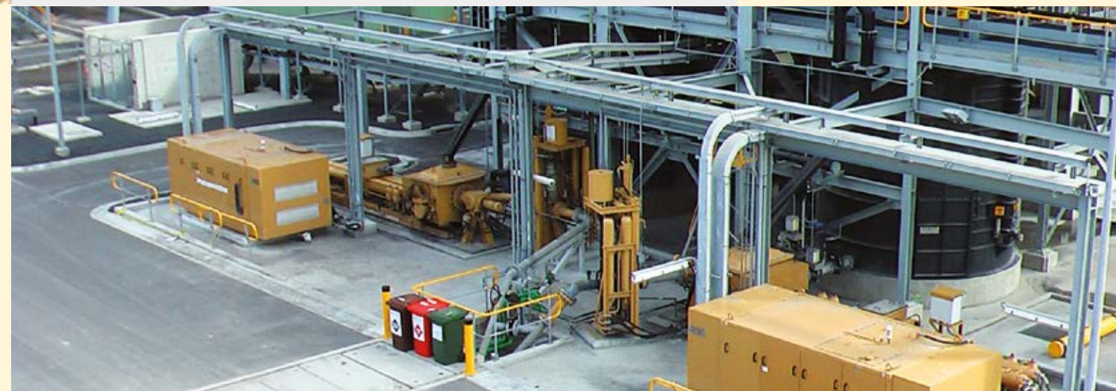
A KOS 25100 pump installation (Kogan Creek, Australia) for fly and bottom ash
