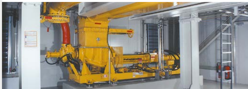
Co-incineration of sewage sludge in the coal-fuelled power plant of Zolling (Germany): KOS 2180
