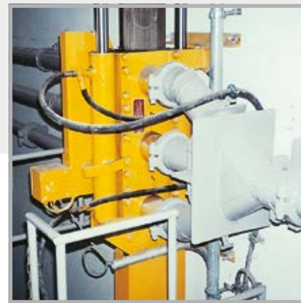
Gate valves for there different delivery lines
