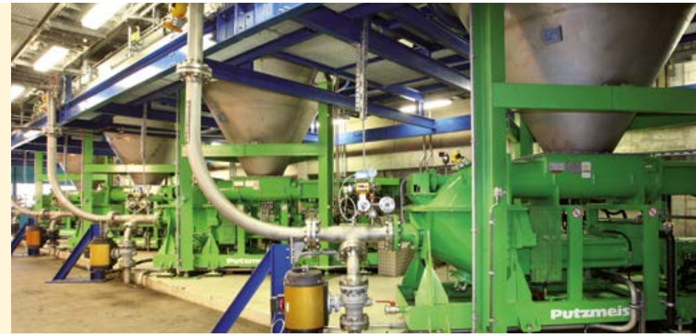
KOS 1050 solids pumps in the ProReno sewage treatment plant in Basel
