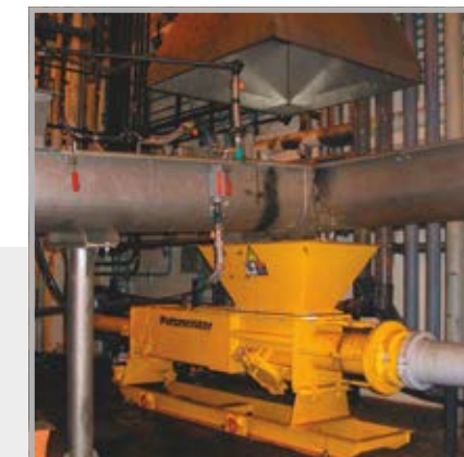
Pumping screenings (Coney Island, New York)
