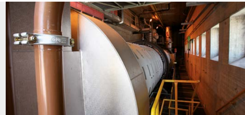
Erzo Oftringen sewage treatment plant (Switzerland): rotary kiln for the incineration of sewage sludge
