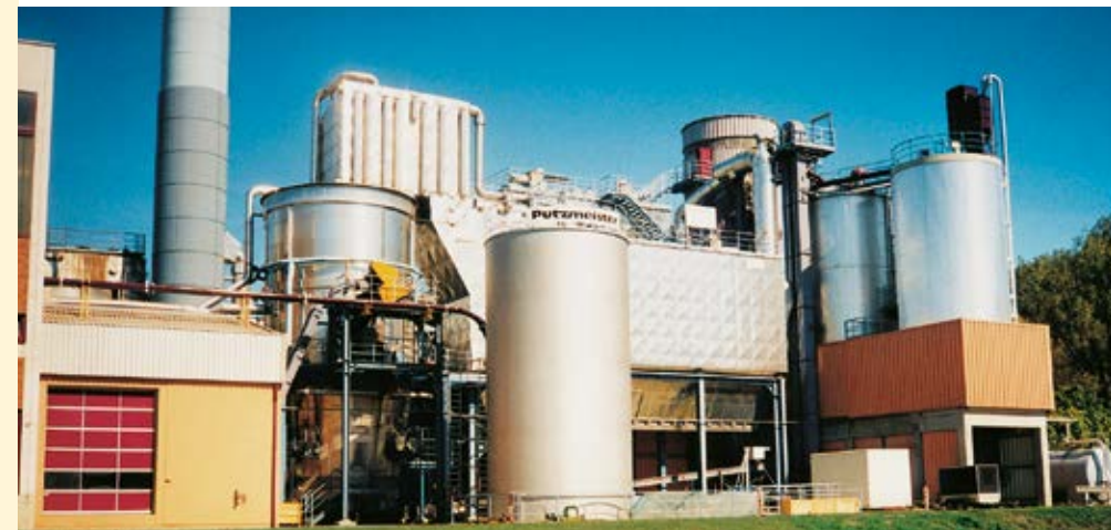
Sewage sludge reception station consisting of reception and storage silos: Incineration of foreign sludge at the main wastewater treatment plant of Stuttgart-Mühlhausen
