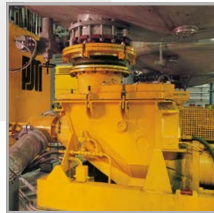
Above: Coal sludge reception system in a power plant Below: KOS 2180 coal transportation pump for longdistance coal delivery
