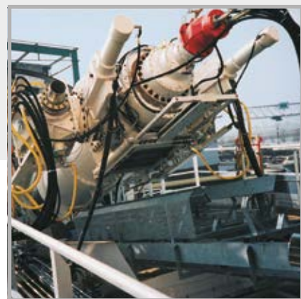
Auger conveyor with two muck pumps of type KOS 1480 (Botlek tunnel, Netherlands)
