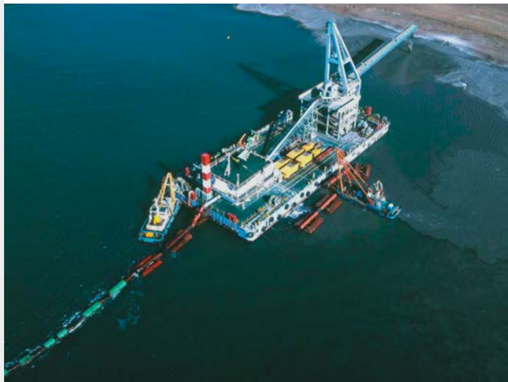
On the Japanese coast line, three huge KOS 25100 and 25200 piston pumps are pumping silt out of the sea for land reclamation. The Nagoya is now located on this new artificial island.
